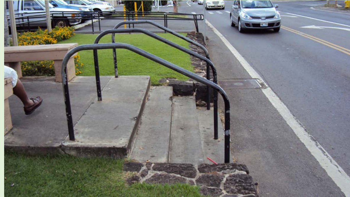
Current stairs and ramp at Jack in the Box on makai side of the Highway
