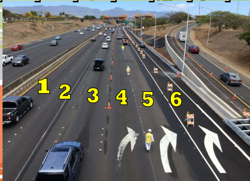
H1 Westbound, next to Waipahu Off-Ramp
