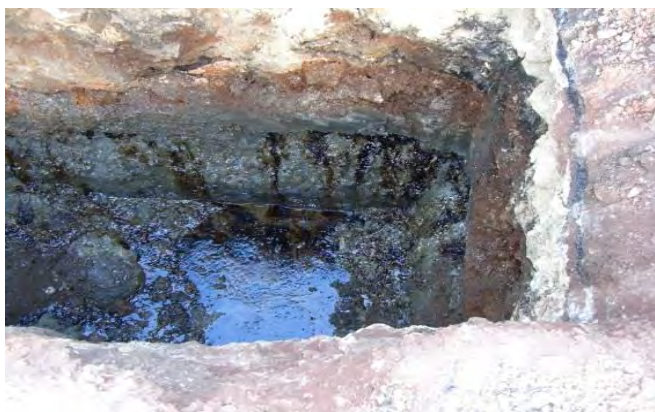
Free product seeping from the side of an excavation.
