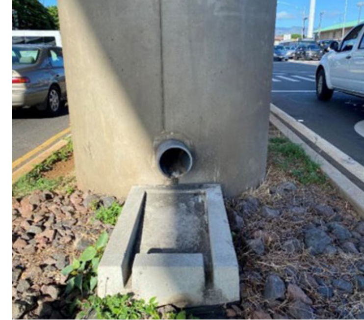
Splashblock located along HART, Daniel K. Inouye International Airport Source: Hawaii DOT
