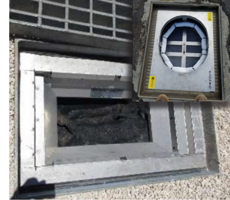
Drain Inlet Insert at Maintenance Baseyard (right) and Drain Inlet Insert at Elliott Street Parking Lot (left), Daniel K. Inouye International Airport Source: Hawaii DOTA
