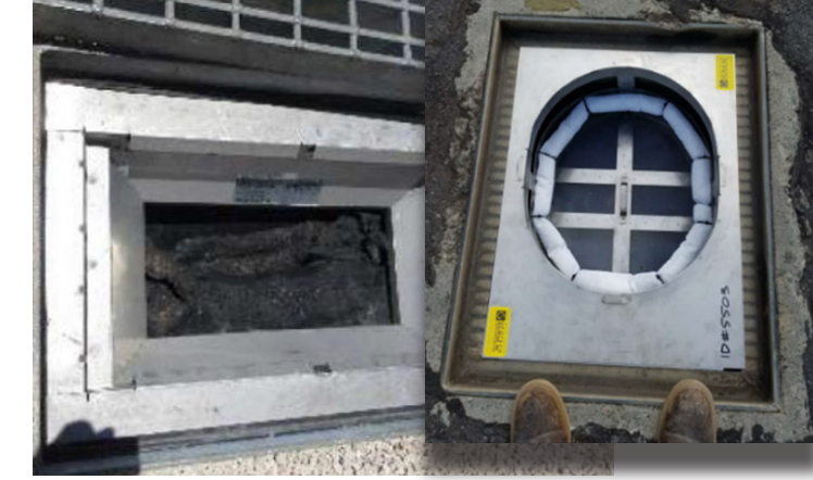
Drain Inlet Insert at Maintenance Baseyard (right) and Drain Inlet Insert at Elliott Street Parking Lot (left), Daniel K. Inouye International Airport Source: Hawaii DOTA
