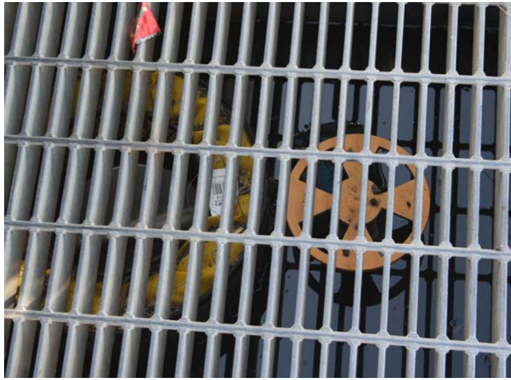
Photograph 13: Safe drain located in the fueling area.
