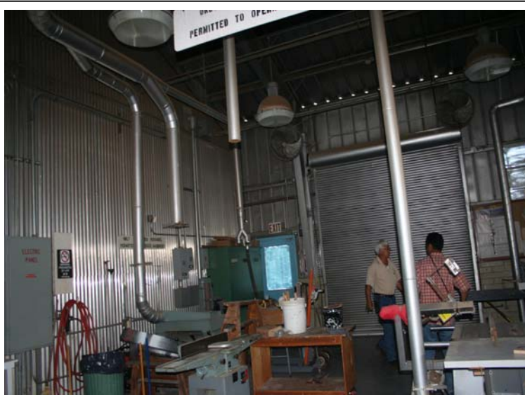
Photograph 18: Interior of the Carpentry Shop. Visible piping is a part of the sawdust vacuum system.
