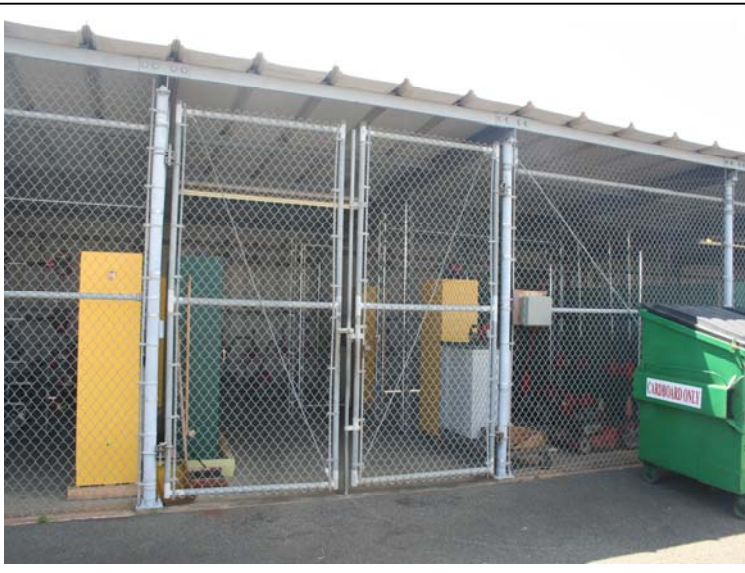
Photograph 21: Small equipment and flammable storage lockers in the shed near the fueling area.
