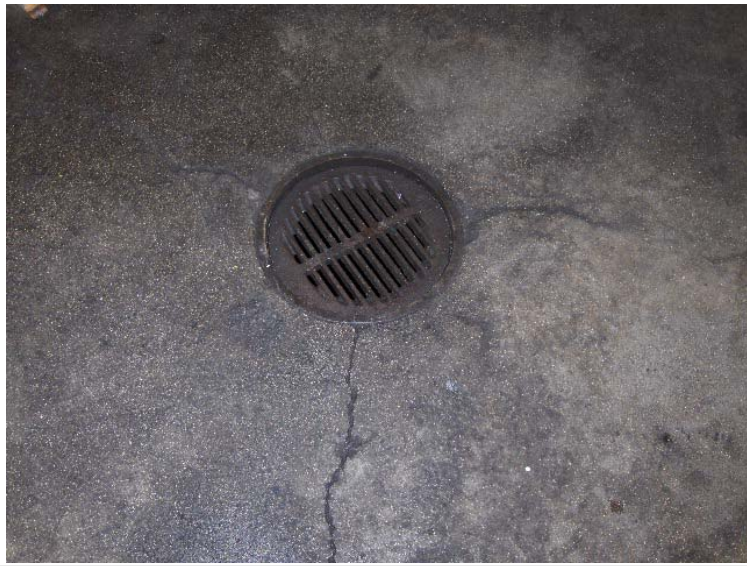
Photograph 4: Floor drain in the maintenance shop to the oil water separator (03907)
