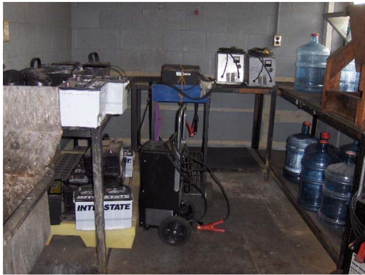
Photograph 10: Battery charging room within the maintenance shop.
