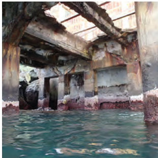
4. Hole in pier deck at shoreward end of trestle.
