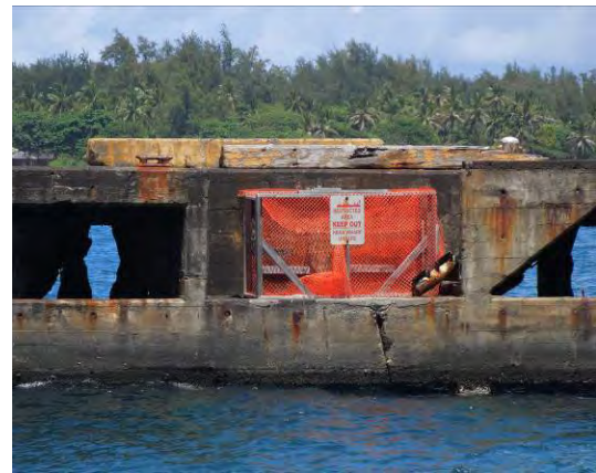
Photo 65. Damaged SW side of Deck 3-28-13
