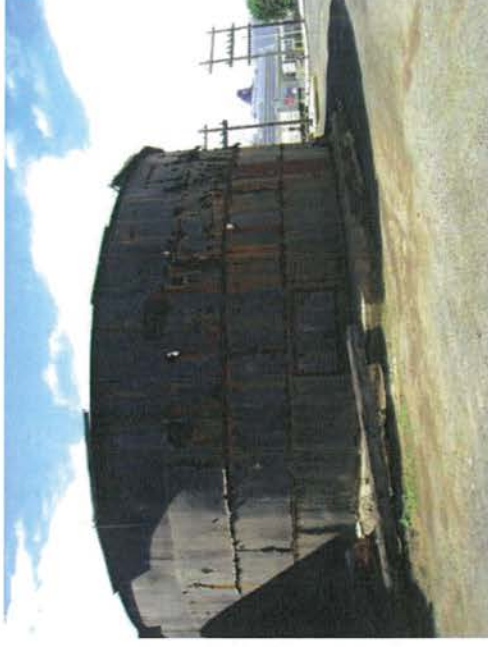
Figure 2: Molasses Storage Tank (1)
