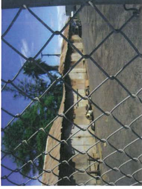
Figure 15: Truck Repair Bays (8) front elevation, partially collapsed
