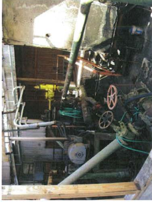
Figure 8: Pump-House (4) adjacent to Tank (3)
