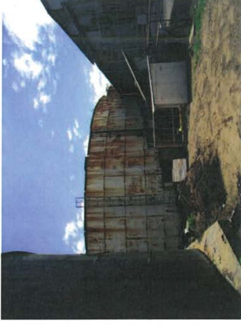
Figure 5: Molasses Storage Tank (3)
