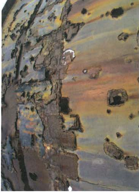
Figure 3: Close-up of exterior rust at Molasses Storage Tank (2)
