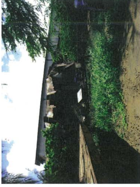
Figure 16: Truck Repair Bays (8) rear elevation, partially collapsed
