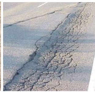
Wheel Track Rutting
